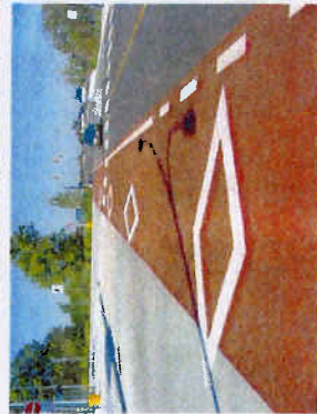
Integral Color Asphalt Ped/Bike Pathway (At palm-lined Upper Trail)
